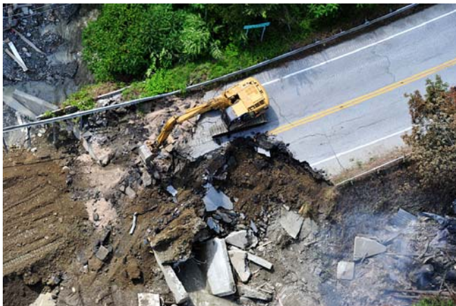
WASHOUT NEAR PITTSFIELD
